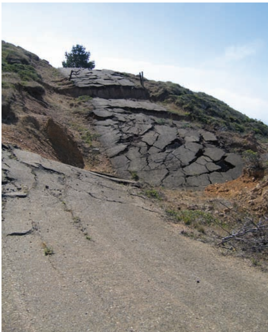
Road in a Marin Headlands mélange zone being slowly destroyed as the land slides from under it
