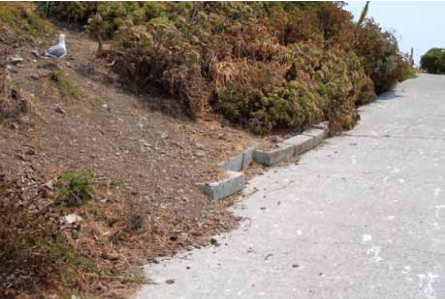
Dilapidated retaining wall and spilling dirt at West Road Terraces, summer
