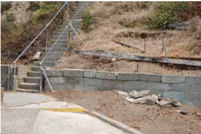
Deteriorated retaining wall at base of recreation yard stairs, summer
